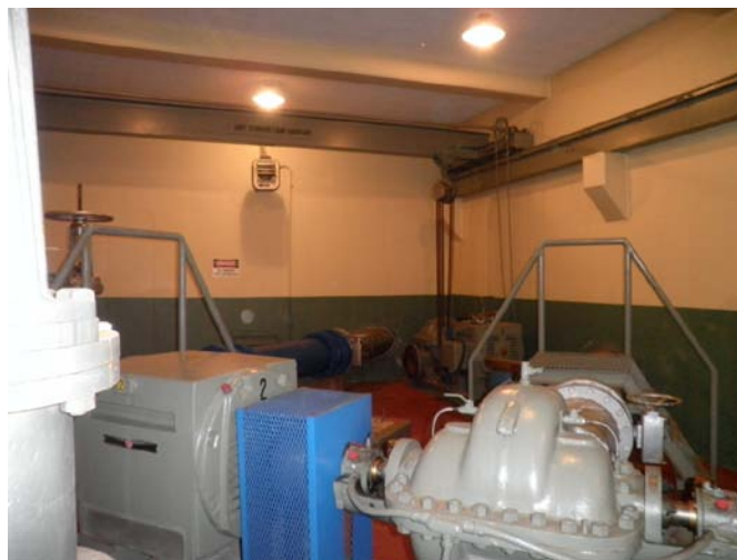
Figure 6 – North City Pump Station Interior
