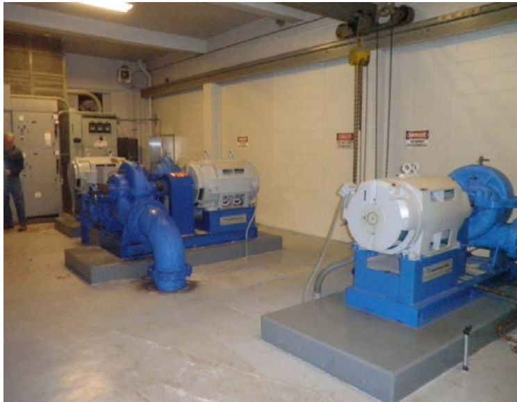
Figure 8 – Foy Pump Station Interior
