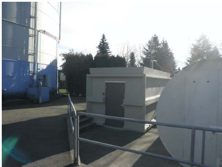
Figure 10 – Dayton Pump Station Exterior
