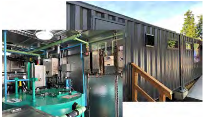
Example of a small anaerobic digester in Redmond (Photo courtesy of Impact BioEnergy, Inc.)
