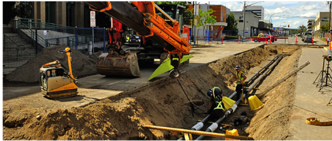
Figure 3 — Prince George District Energy System The downtown renewable energy system connects numerous buildings through the downtown, providing them with hot water heat.
