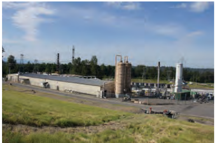
The Bio Energy Washington plant at Cedar Hills landfill converts landfill gas to pipeline quality gas
