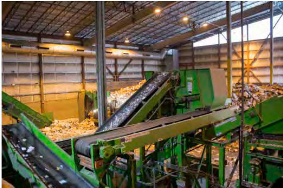
Recology CleanScapes materials recovery facility
