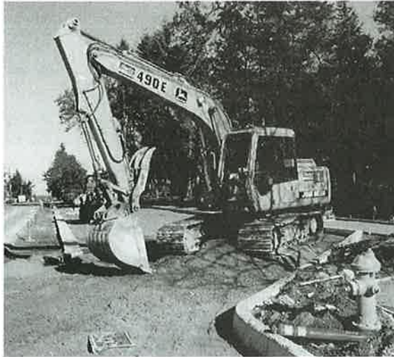
Construction of parking improvements and additions underway at the Shoreline Pool is one of the projects listed in the 1999 Capital Improvement Program.
