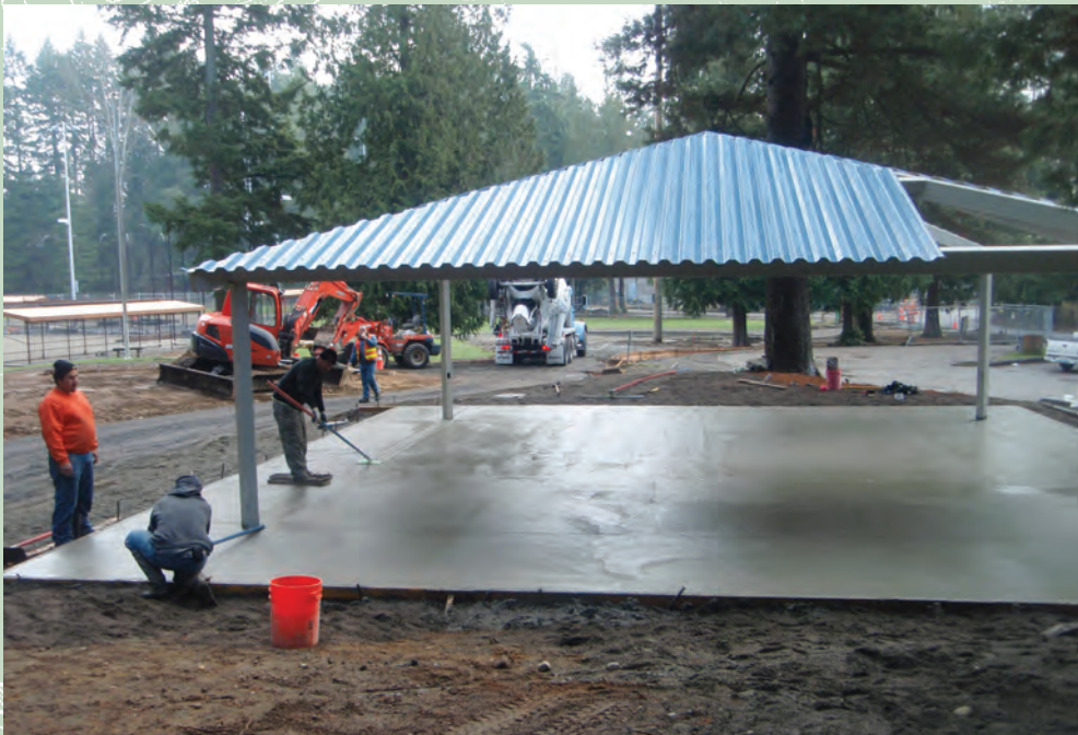
The construction crew works on the concrete base for the Hamlin Park picnic shelter before benches and tables are installed.
