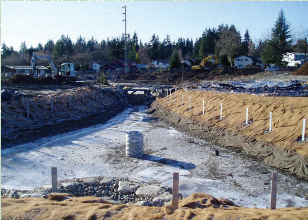
Looking southwest from the main pathway towards Meridian Avenue shows the footing for the projects public art piece, "Rain Tree" within the storm water detention pond at Cromwell Park. The public art piece will celebrate water in our environment. The storm water improvements at Cromwell are designed to reduce potential flooding impacts at Ronald Bog and further downstream.
