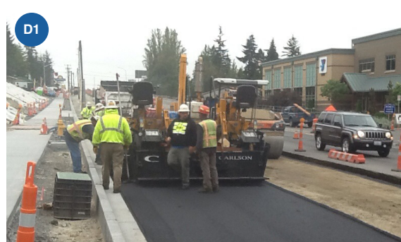
D1. Paving the first lift of the future southbound business access and transit lane
