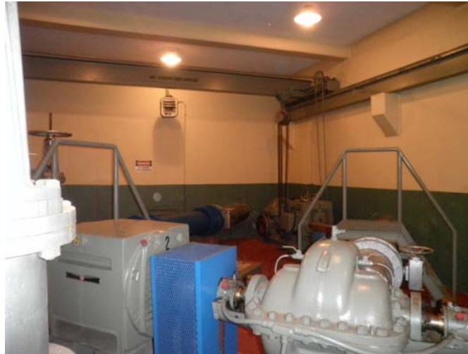
Figure 6 – North City Pump Station Interior
