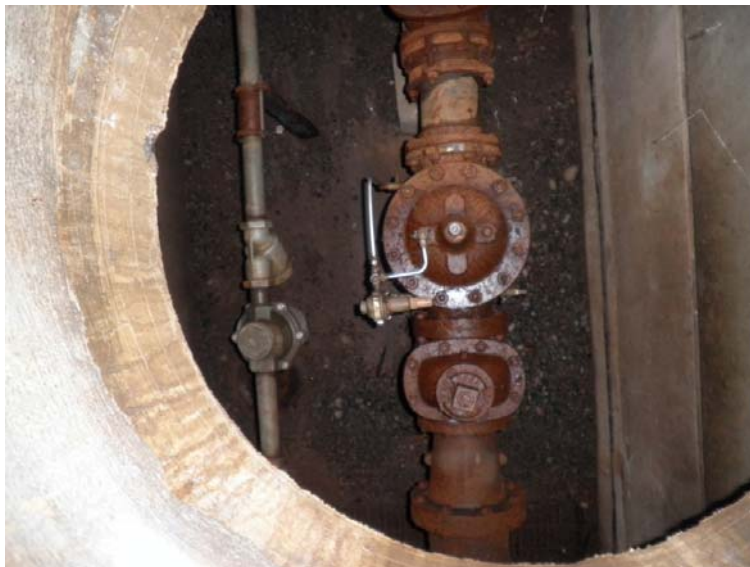
Figure 14 – Pressure Reducing Valve, 9th Ave NW & Innes Arden Way
