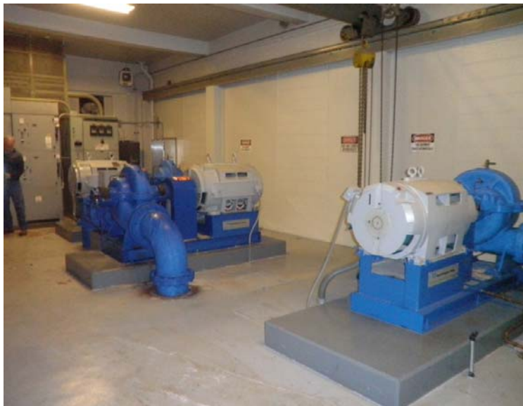
Figure 8 – Foy Pump Station Interior
