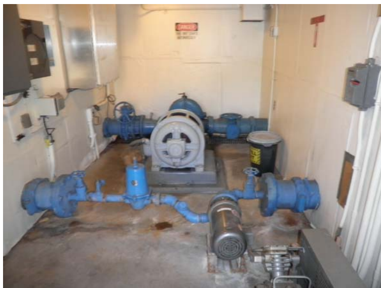
Figure 11 – Dayton Pump Station Interior
