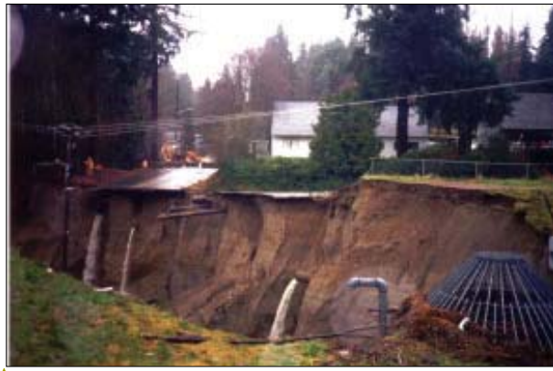
Holiday Blast Storm Sinkhole - Shoreline
