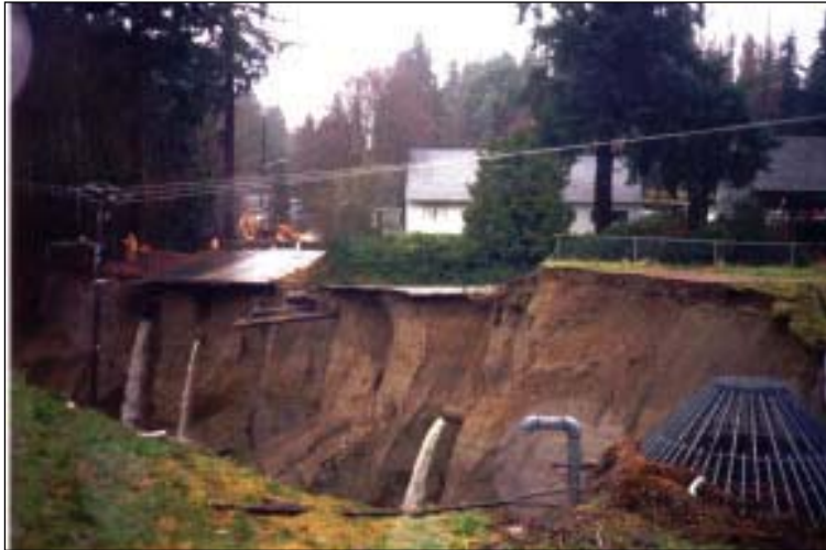
Holiday Blast Storm Sinkhole - Shoreline
