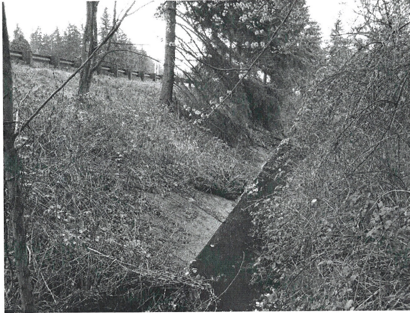
Photo 3, facing southward, downstream, showing a typical channel section.
