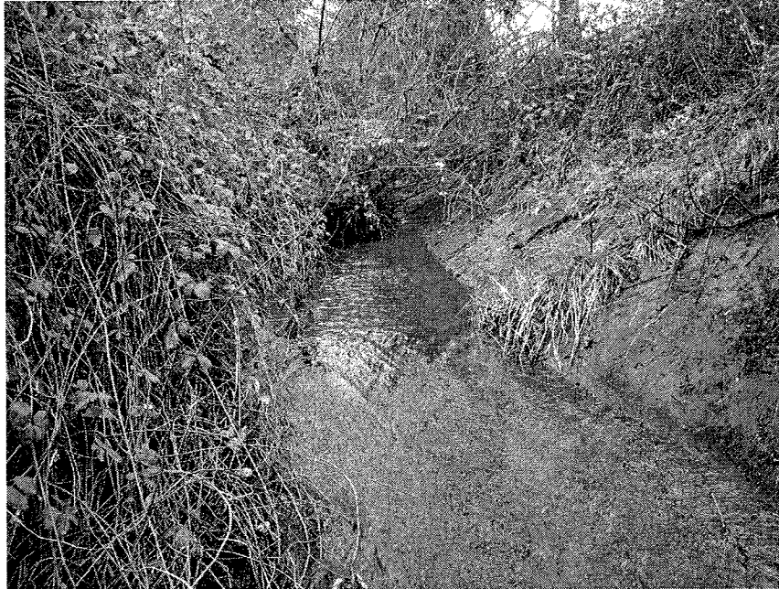
Photo 1, Thornton Creek concrete channel, facing northward, upstream from near the I-5 culvert entrance.
