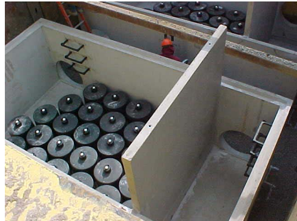
Figure 10: Stormfilters in Catch Basin Insert (Image from Contech)
