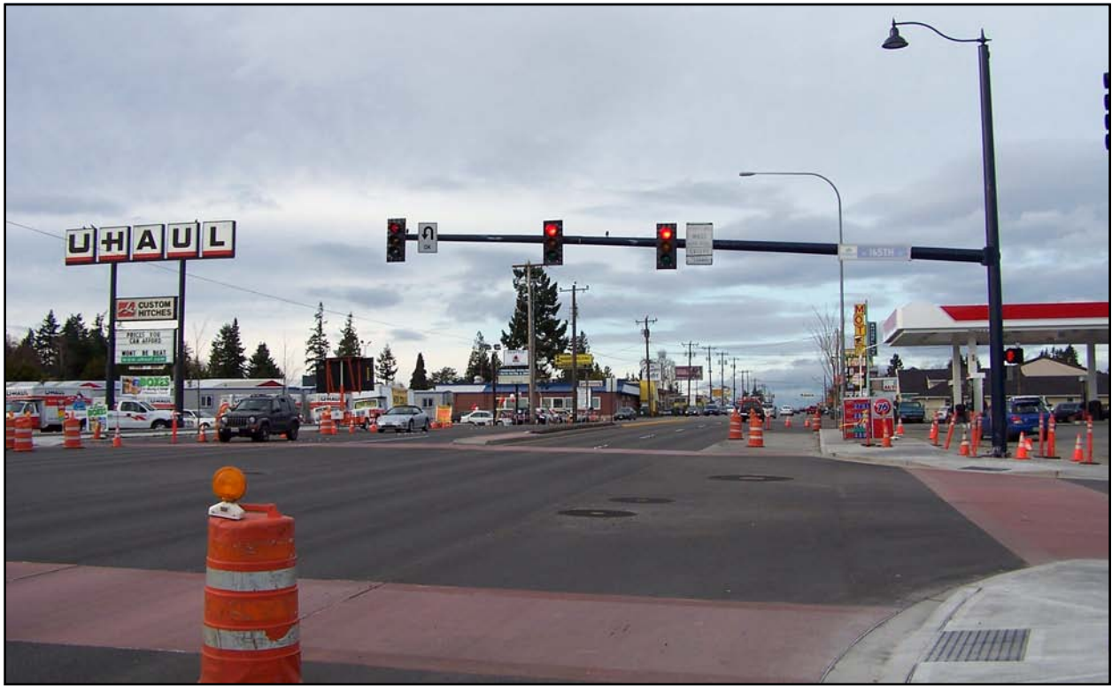
Viewpoint 3: View North towards Project. Facing north towards entrance of project corridor near N 165th Street within Landscape Unit 1.
