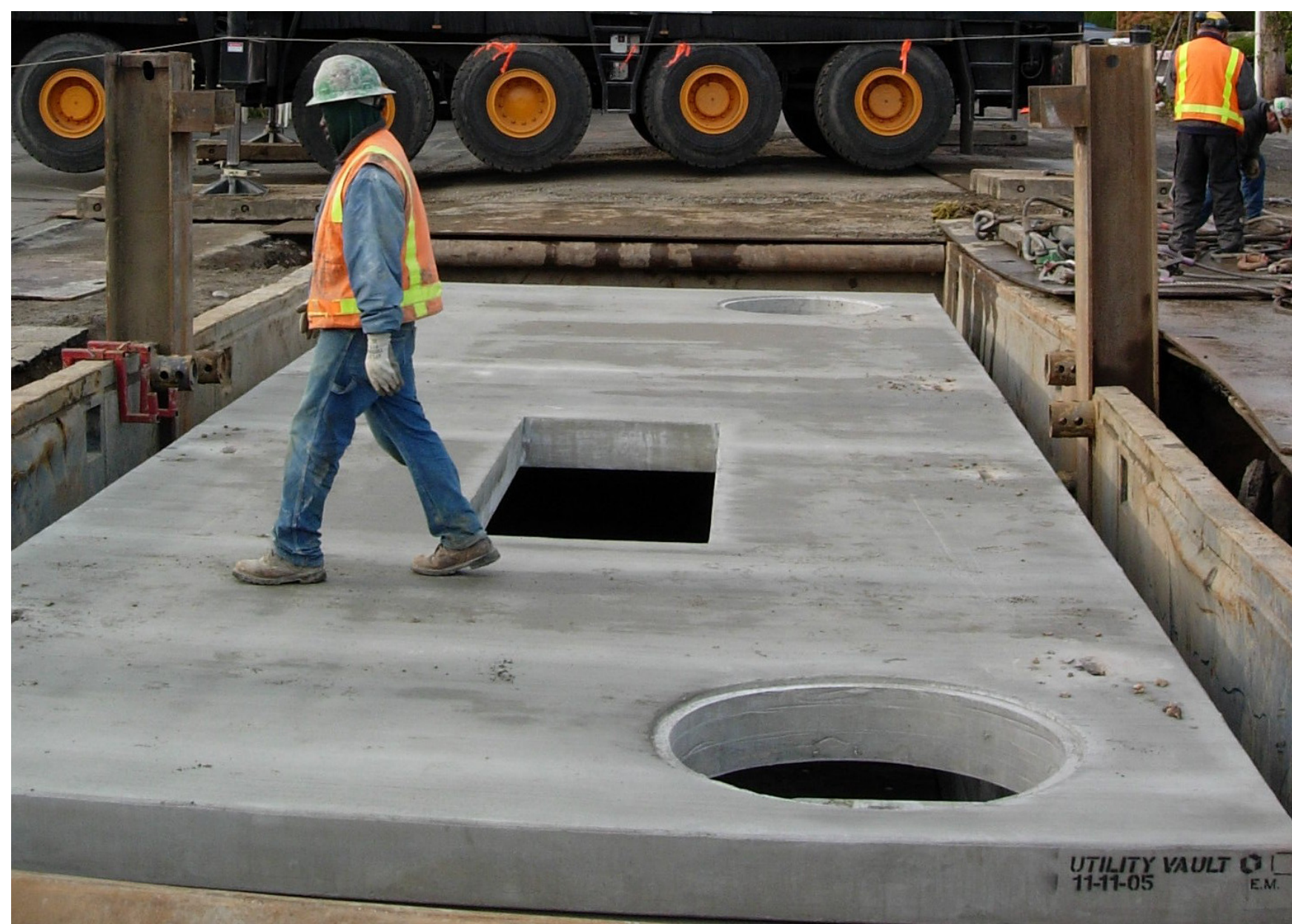
Stormwater Treatment Vault
