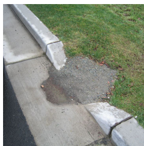
sediment buildup at curb cut
