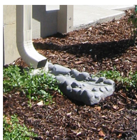
downspout splash block
